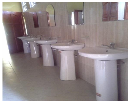
Wash hand basins inside the toilets
